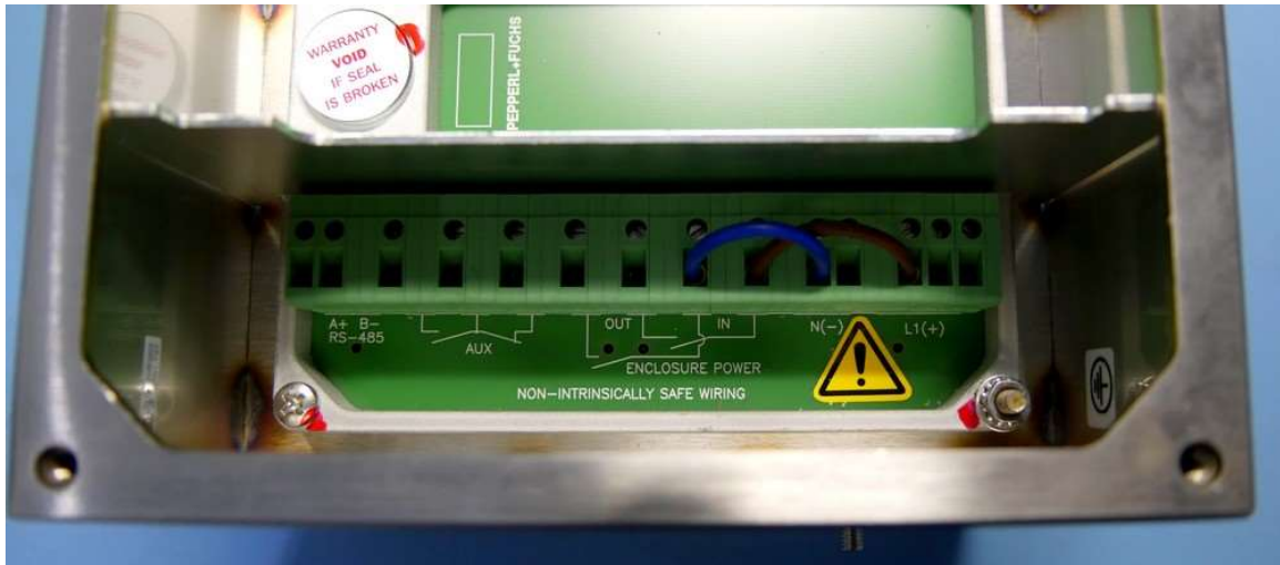
Figure 206. Jumpers placement for powering the main supply switch in purge controller.
